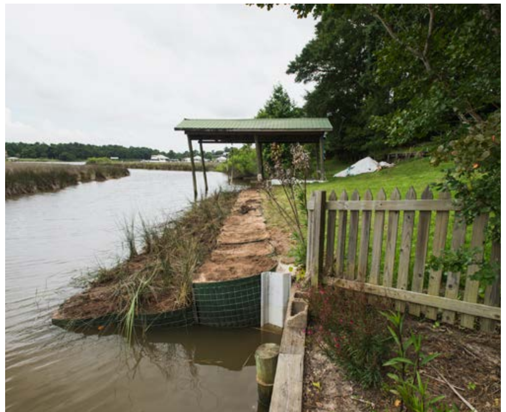
Top: Construction of the first private living shoreline. (Photo by Mary Kate Brown, The Nature Conservancy)
