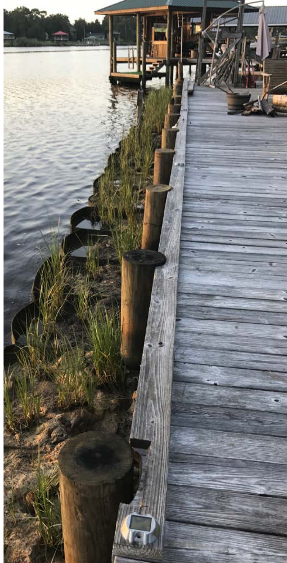
Previous page and right: Completed bulkhead retrofit with marsh grasses. (Photo by Jacob Blandford, The Nature Conservancy)
