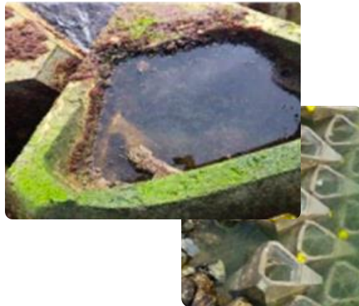
Pilot study of EConcrete Coastalock armor units in the San Diego port 88
