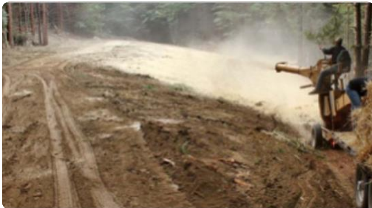
Seeding and mulching (suing a straw blower) of an exposed area from a decommissioned road
